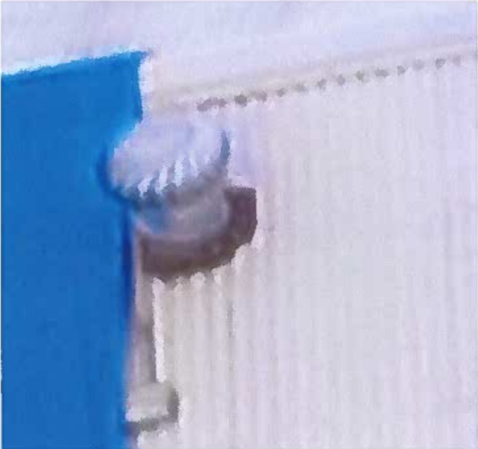
Typical roof air ventilator
